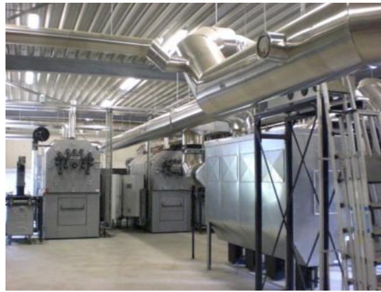
Biomass plant (district heat)
